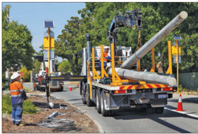
• Poles will disappear when South Freqo's power goes underground.
